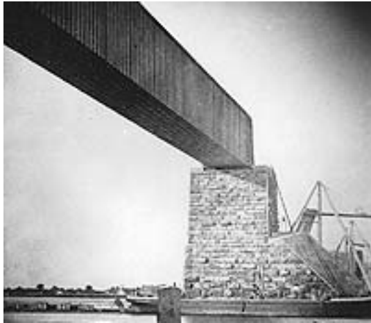
The Victoria Bridge under construction, in 1859 Centre tube and No. 13 pier, Victoria Bridge, Montreal, QC, 1859, photographer: William Notman. Notman Photographic Archives, McCord Museum of Canadian History, Montreal. VIEW-7013.0
